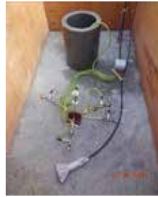
Strain gage rosette and piezometer being installed at Nam Pha Dam, Laos
