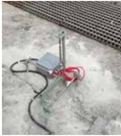
Triaxial jointmeter installed at Teesta III Dam, India
