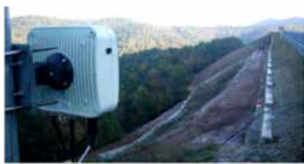
GATEWAY INSTALLED FOR WIRELESS MONITORING
