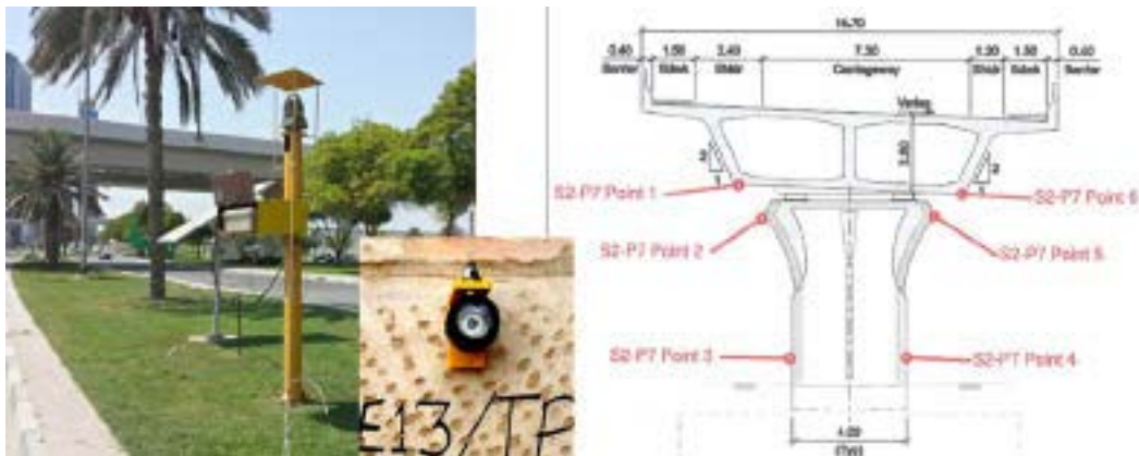
Web-based monitoring of lateral movement and settlement using robotic total stations and prism targets
